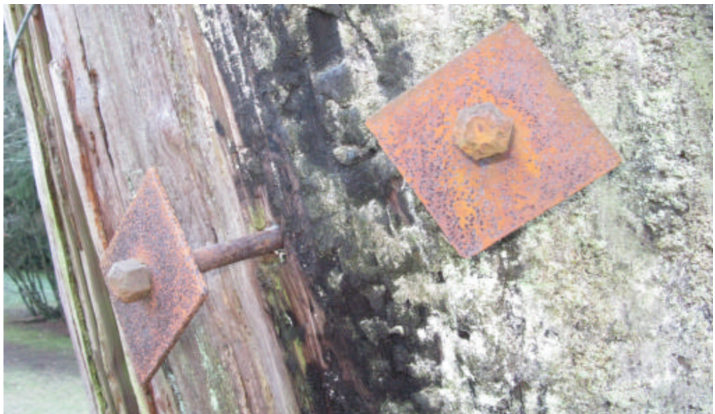
Photo 3: Steel washers and bolts no longer effective
